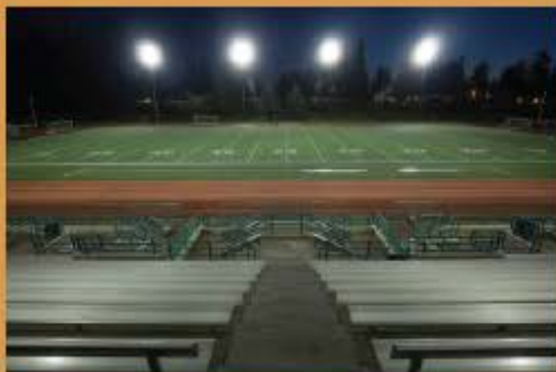
FIELD WITH OLD METAL HALIDE LIGHTING SYSTEM
