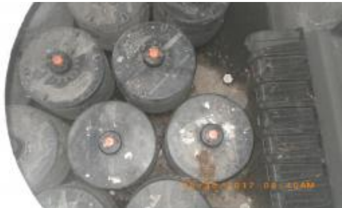
The StormFilter® cartridges in a filter vault
