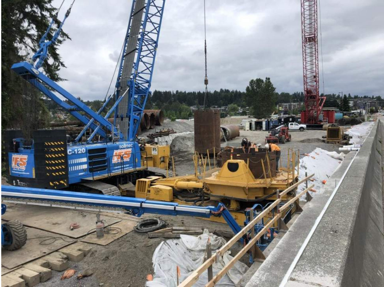
The drilling subcontractor mounts a shaft oscillator platform over the shaft hole and preps a crane for shaft excavation.
