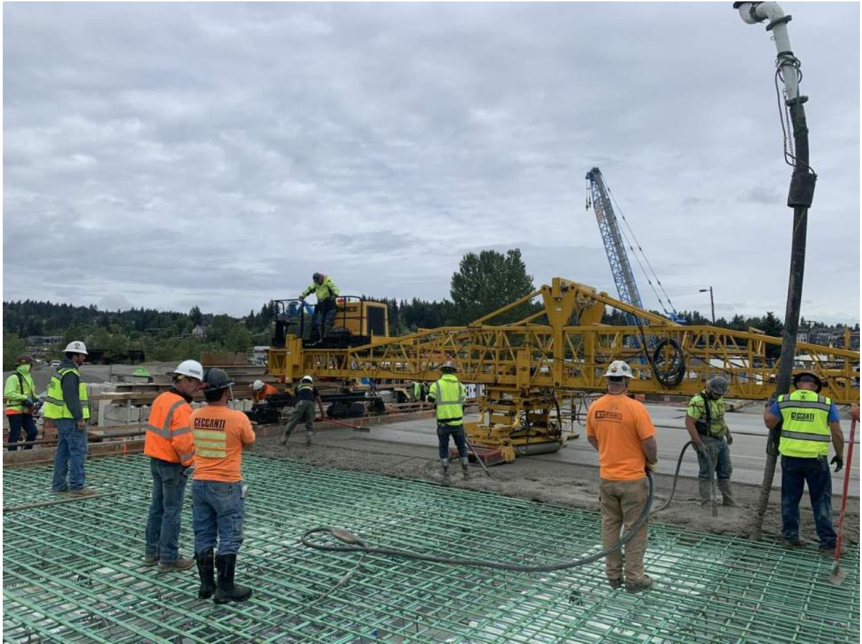
The bridge deck is poured using a concrete pump truck (below the bridge) and a paving machine mounted on rails along either side of the bridge deck extents.
