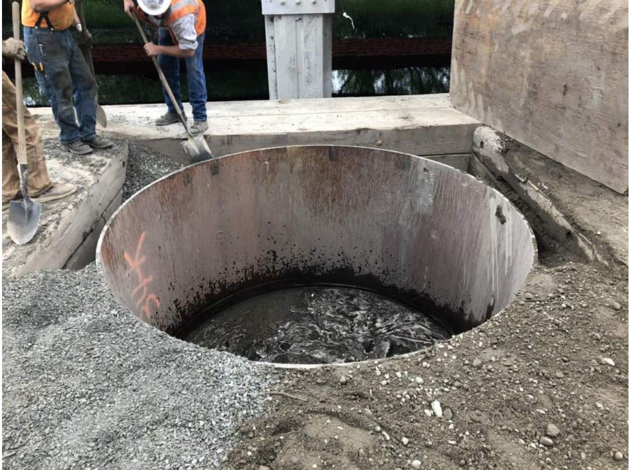
Crews prep the shaft location before beginning main shaft excavation work. The finished shafts will not be visible once the bridge construction is completed.
