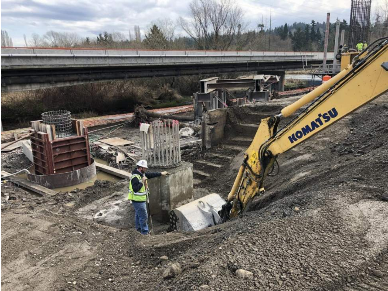
The contractor prepares the tops of the column sections to receive the crossbeam formwork. The tops of the column rebars will extend into the finished crossbeam section.
