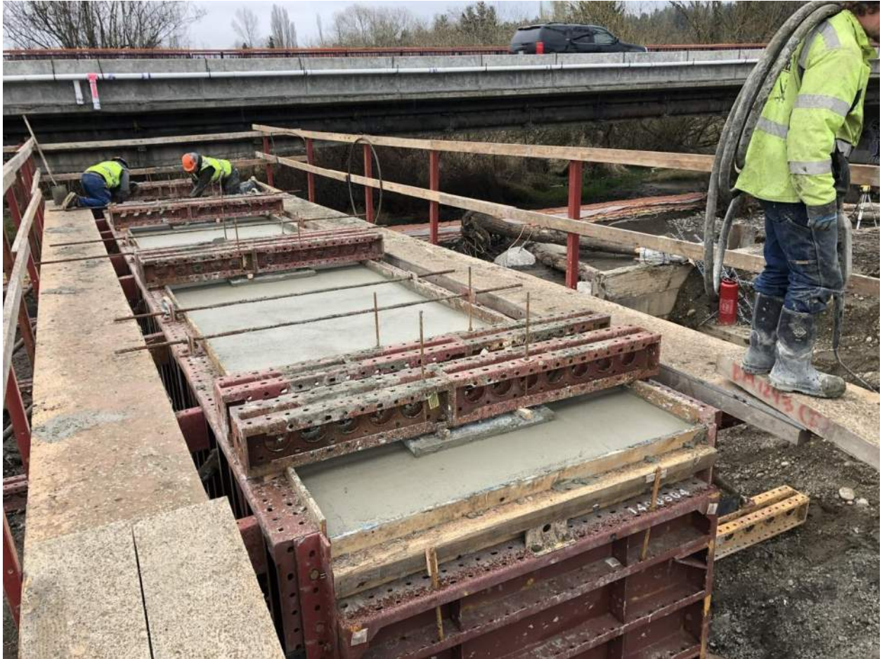
The contractor finishes the top surface of the crossbeam pour and mounts special bearings along the top of the crossbeam to receive each bridge girder.
