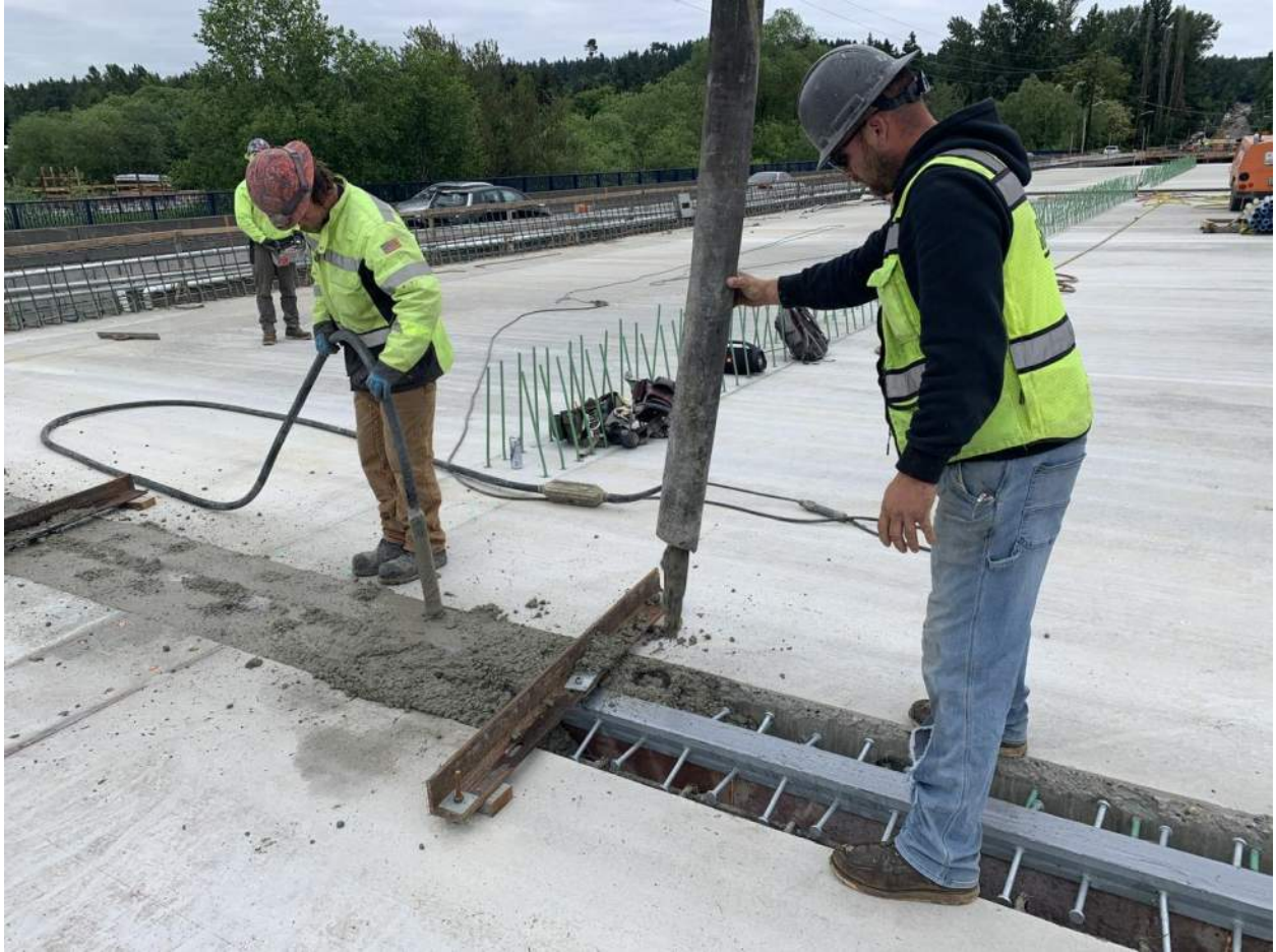
The final pours at the expansion joints on either end of the bridge are completed. Work along the bridge deck will continue until the fully completed bridge is in place and ready for traffic.
