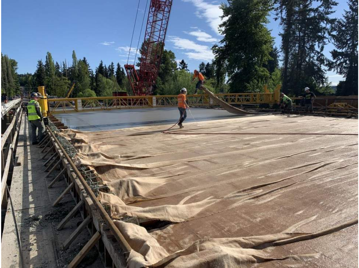
The freshly placed bridge deck concrete is covered with wet burlap and kept wet with soaker hoses to aid in concrete curing (hardening).
