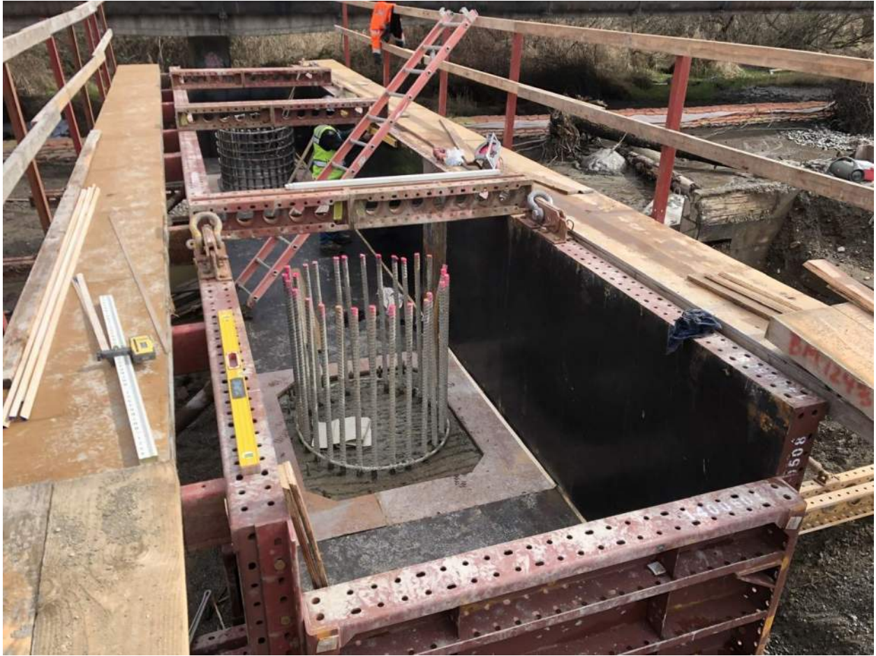
The pier crossbeam formwork is set into position on top of the two column sections at each pier.
