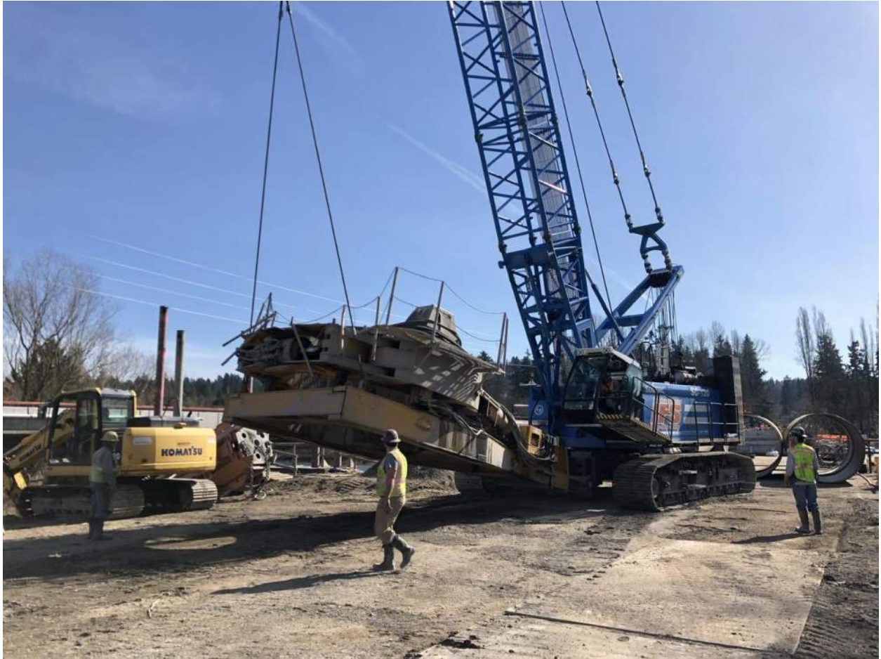
The drilling subcontractor prepares their crane and bridge shaft oscillator platform for foundation shaft installation work.
