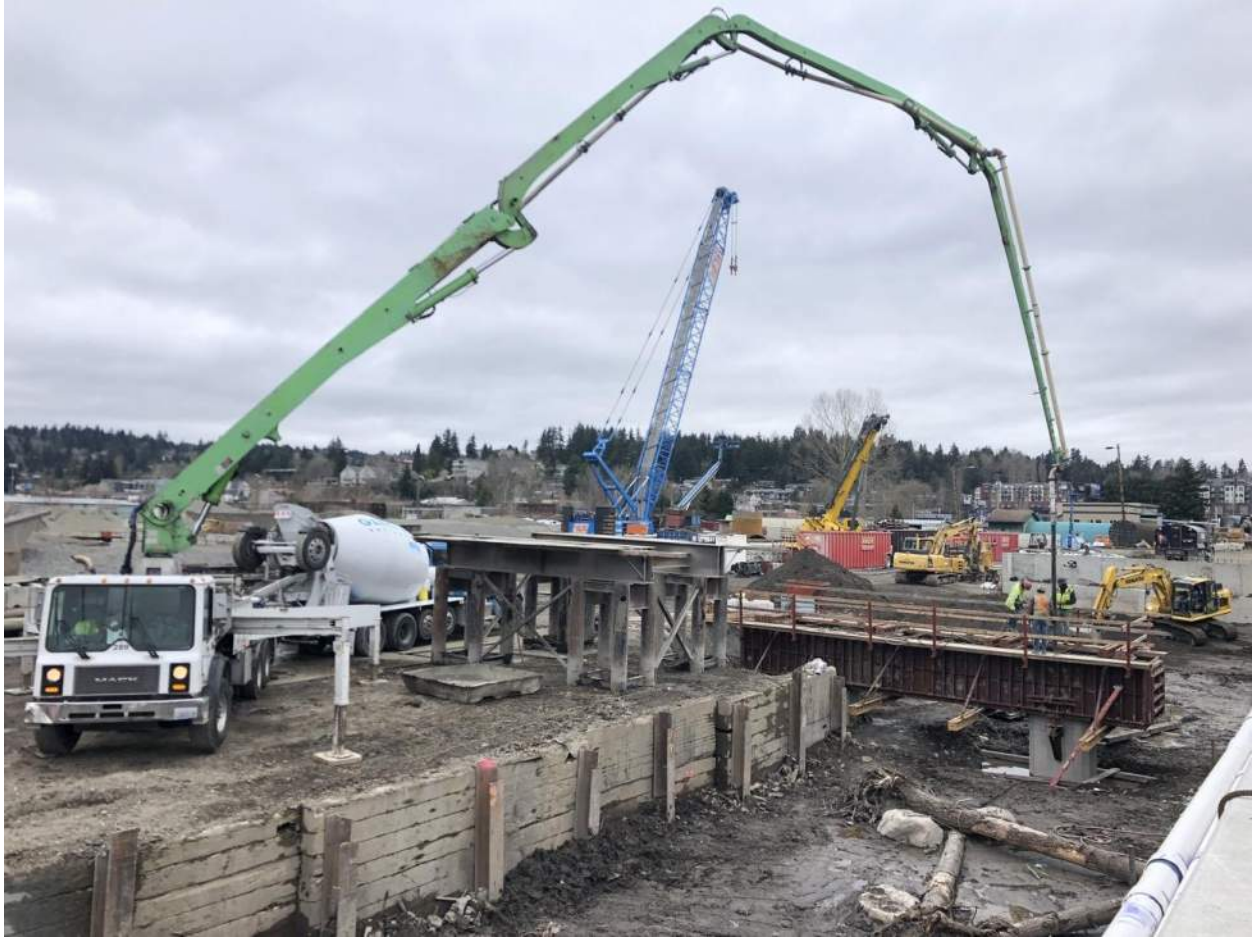
A concrete pump truck is brought in to pour the concrete crossbeam section in the crossbeam formwork.
