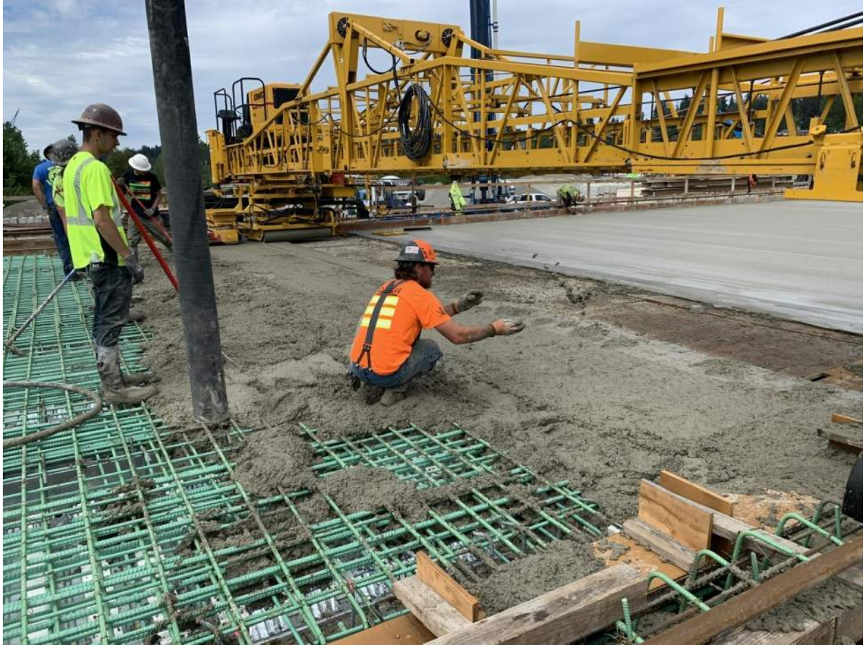
Crews make sure the concrete is placed evenly across the entirety of the deck surface.
