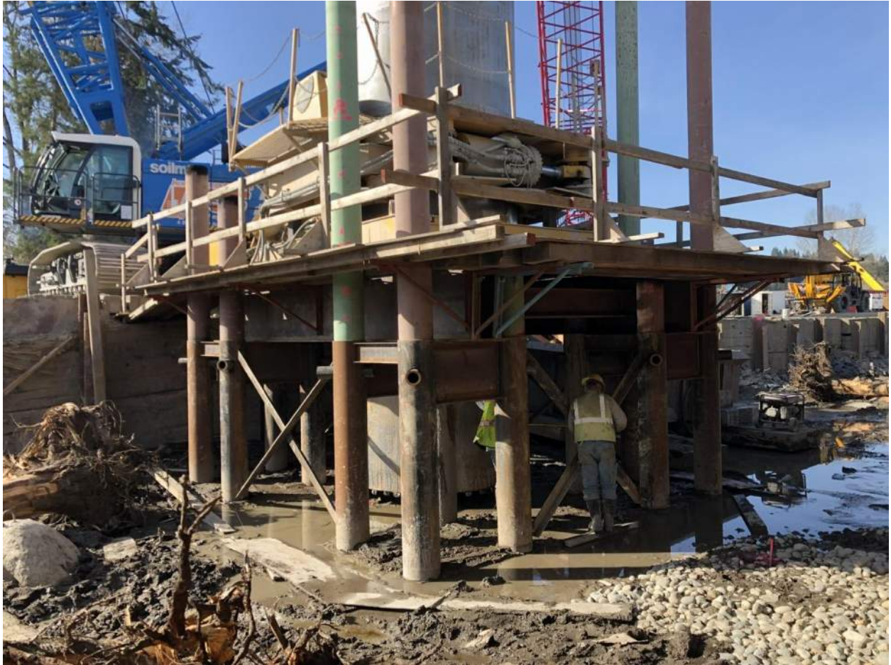
The drilling subcontractor sets up to install the west bridge foundation shaft at Pier 4 using an elevated work platform.
