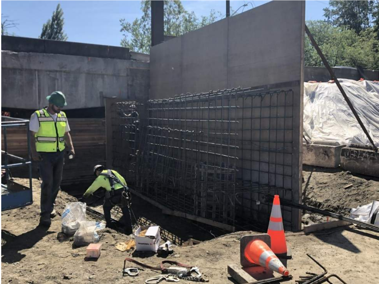
Rebar for the lower part of the abutment section is installed. The abutments are constructed in halves. At Pier 1, the west half-width is being built first.
