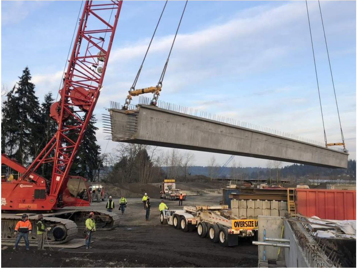
Girders are brought in on specialty trucks and picked by the contractor's large red crane.
