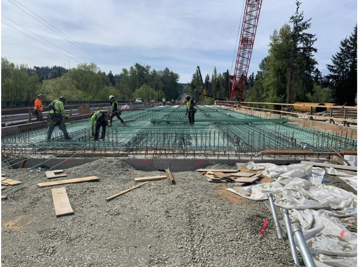
A subcontractor installs rebar for bridge deck reinforcement. These bars are covered with a green protective coating to prevent rusting and corrosion over the life of the bridge.
