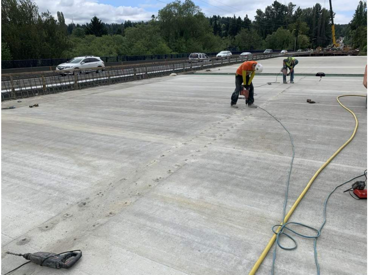
Once deck curing is finished, crews begin drilling into the new deck concrete to prep for new traffic barrier installation.
