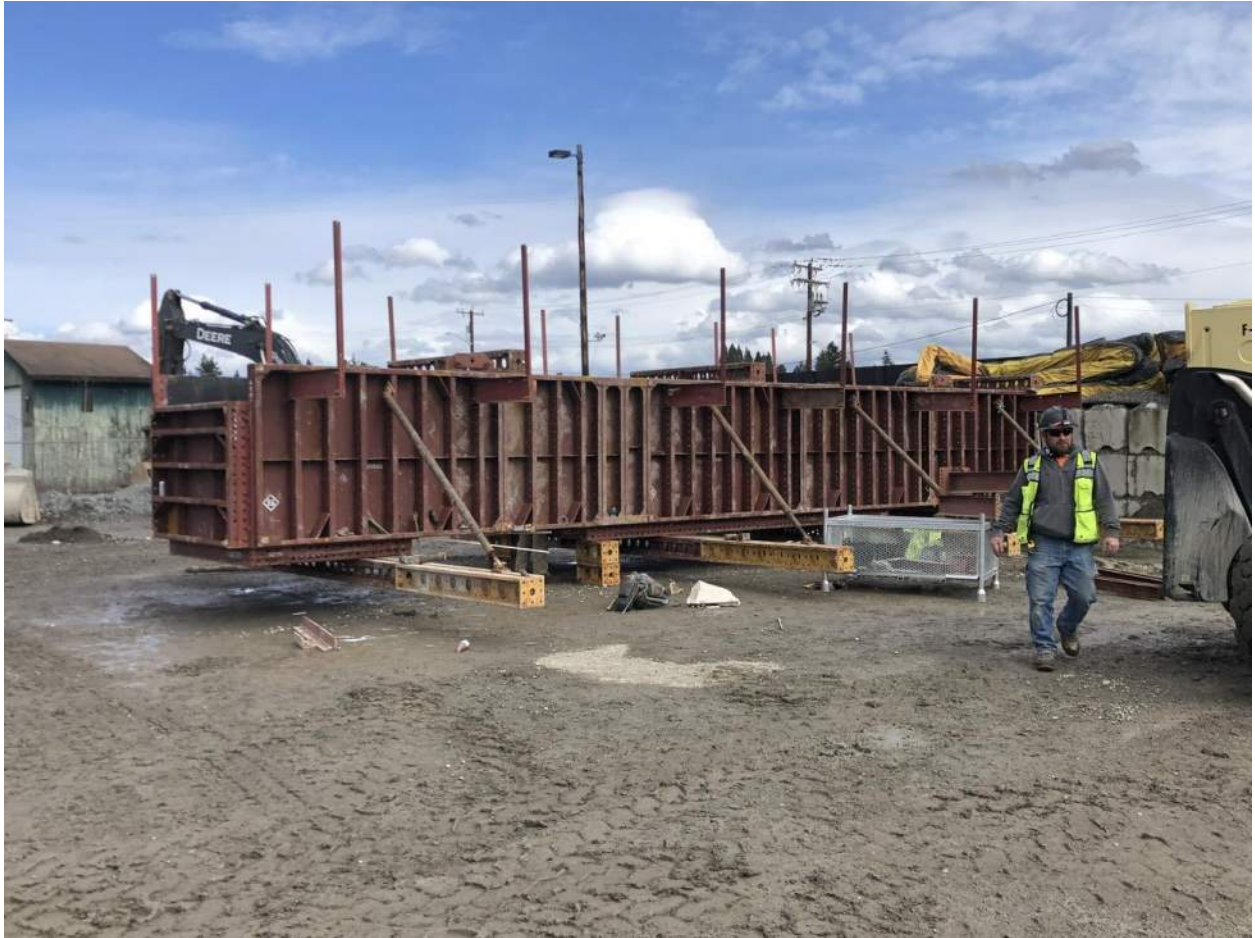
The contractor assembles steel formwork for casting the concrete crossbeams at each of the interior piers along the bridge.
