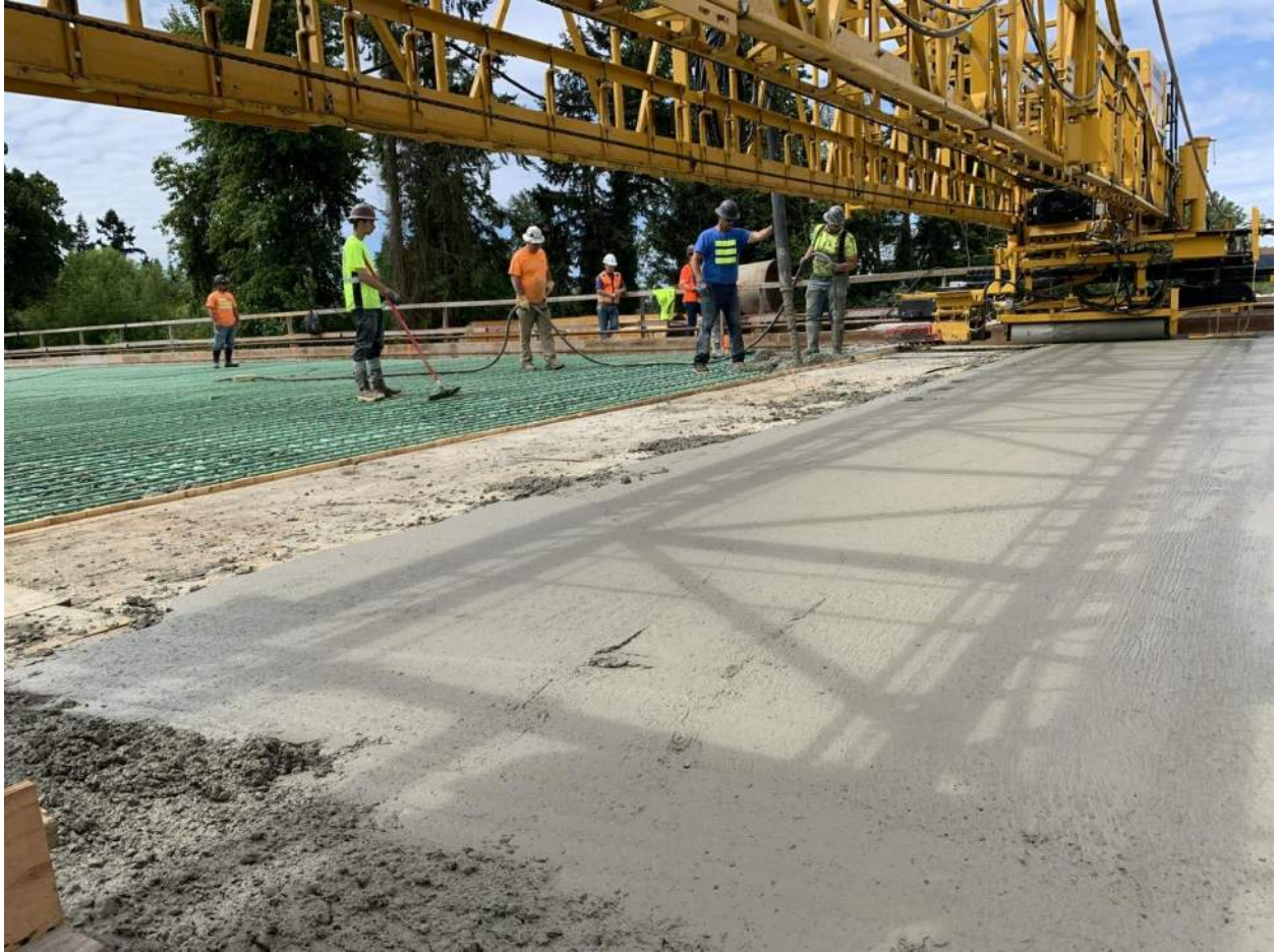
The paving machine has a roller and a brush to finish the top surface of the bridge deck concrete.
