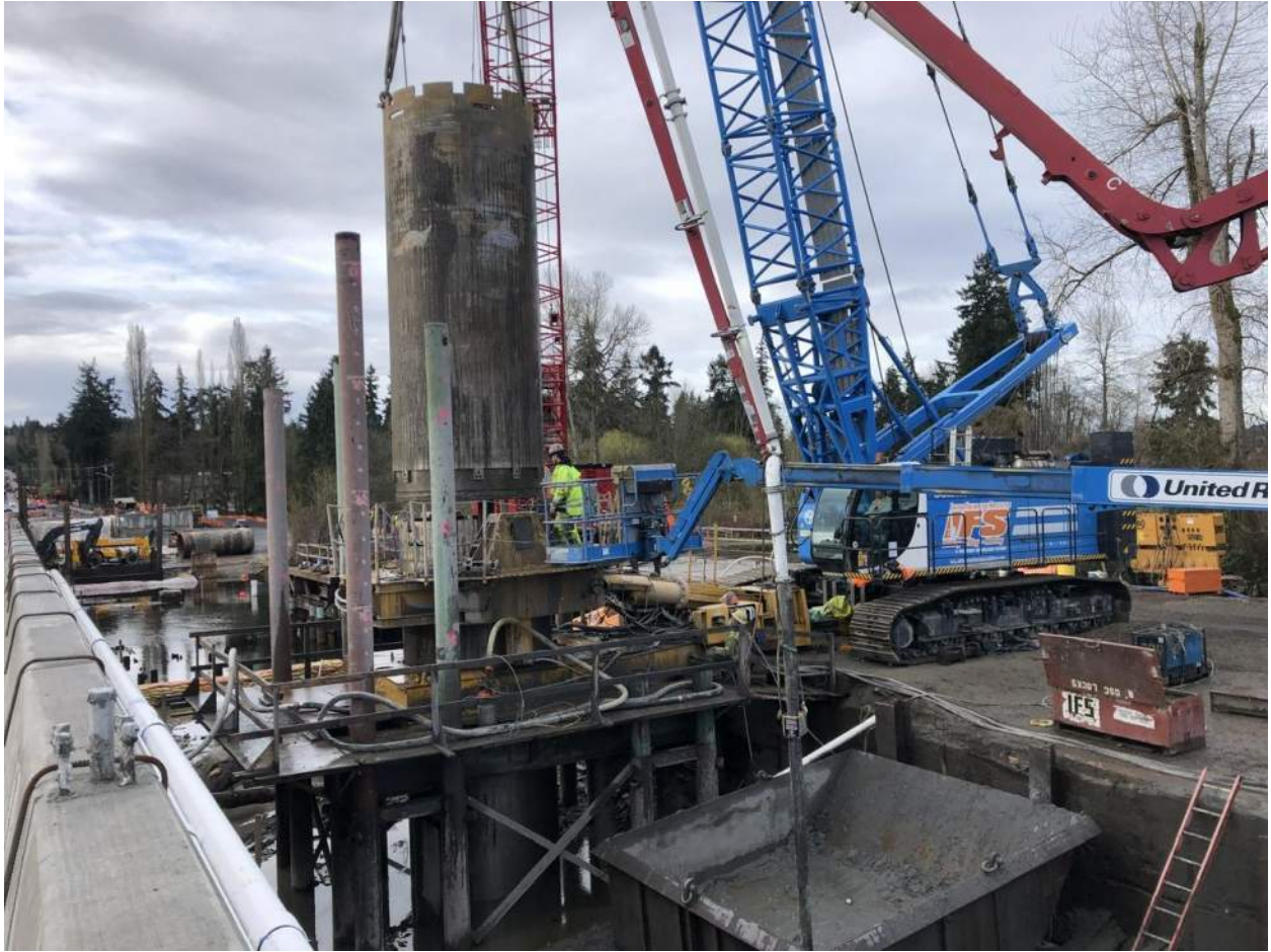
The drilling subcontractor uses temporary steel casing segments and a crane-mounted clamshell bucket to excavate earth from the shaft.
