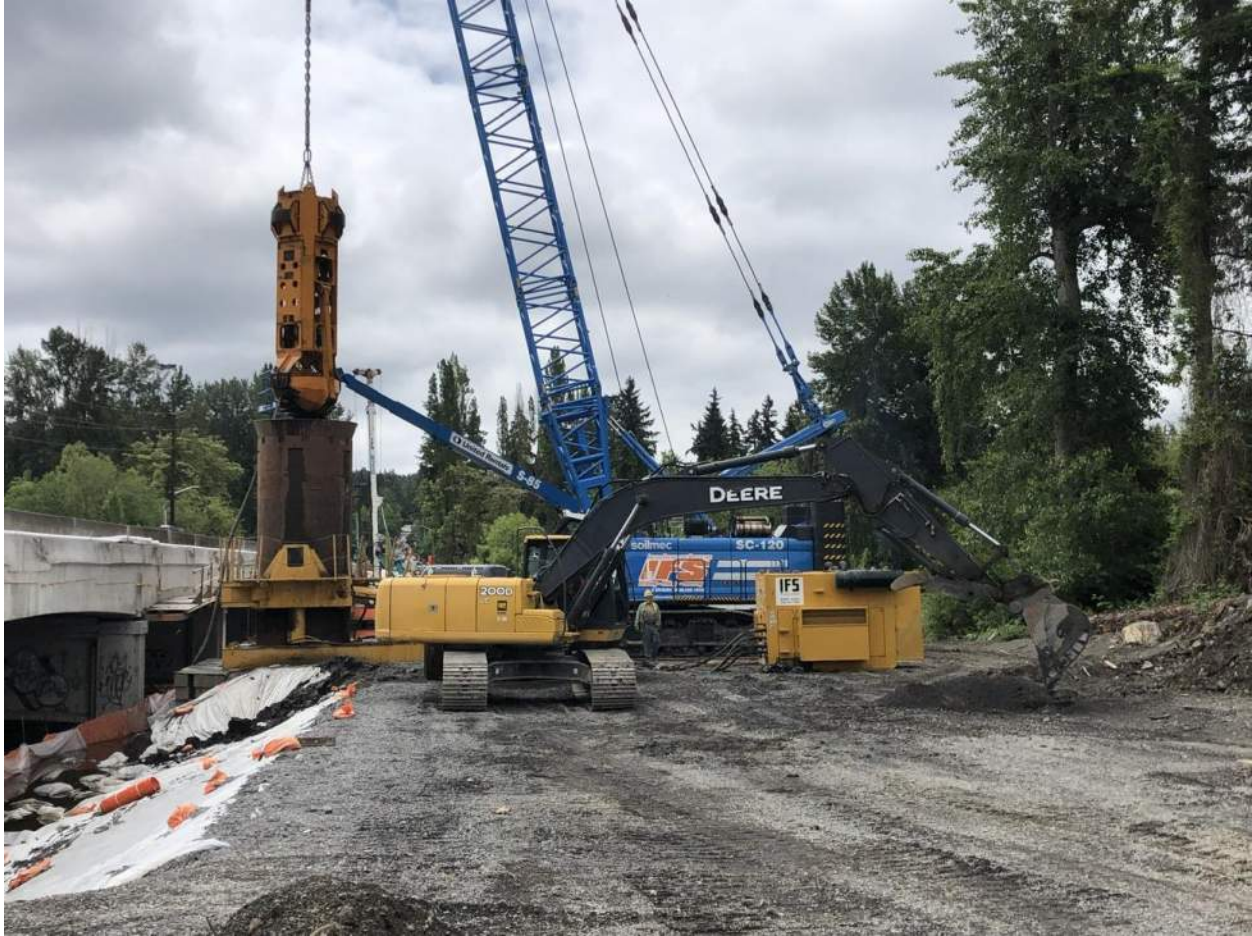
The drilling subcontractor uses a crane-mounted clamshell bucket to excavate earth from the shaft as steel casing segments are slowly lowered ('oscillated') into the ground to bottom-of-shaft depth.
