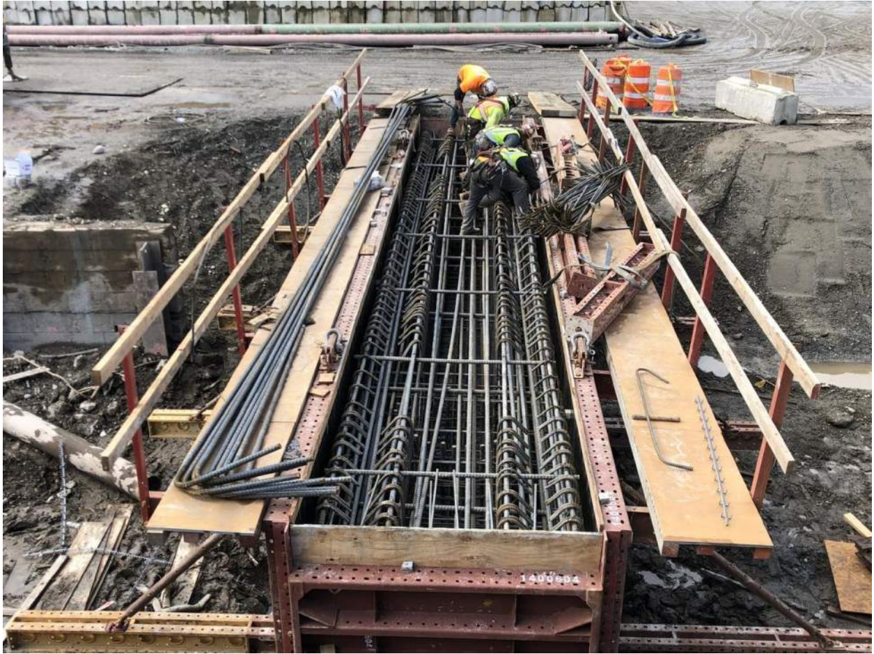
The crossbeam is one of the most heavily reinforced elements of the bridge structure.
