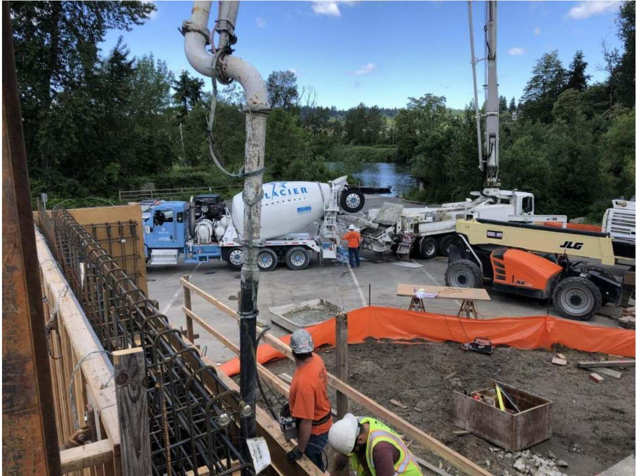
A concrete truck (blue and white) and pump truck are used to pump concrete into the abutment formwork to pour the lower (wider) part of the concrete abutment.
