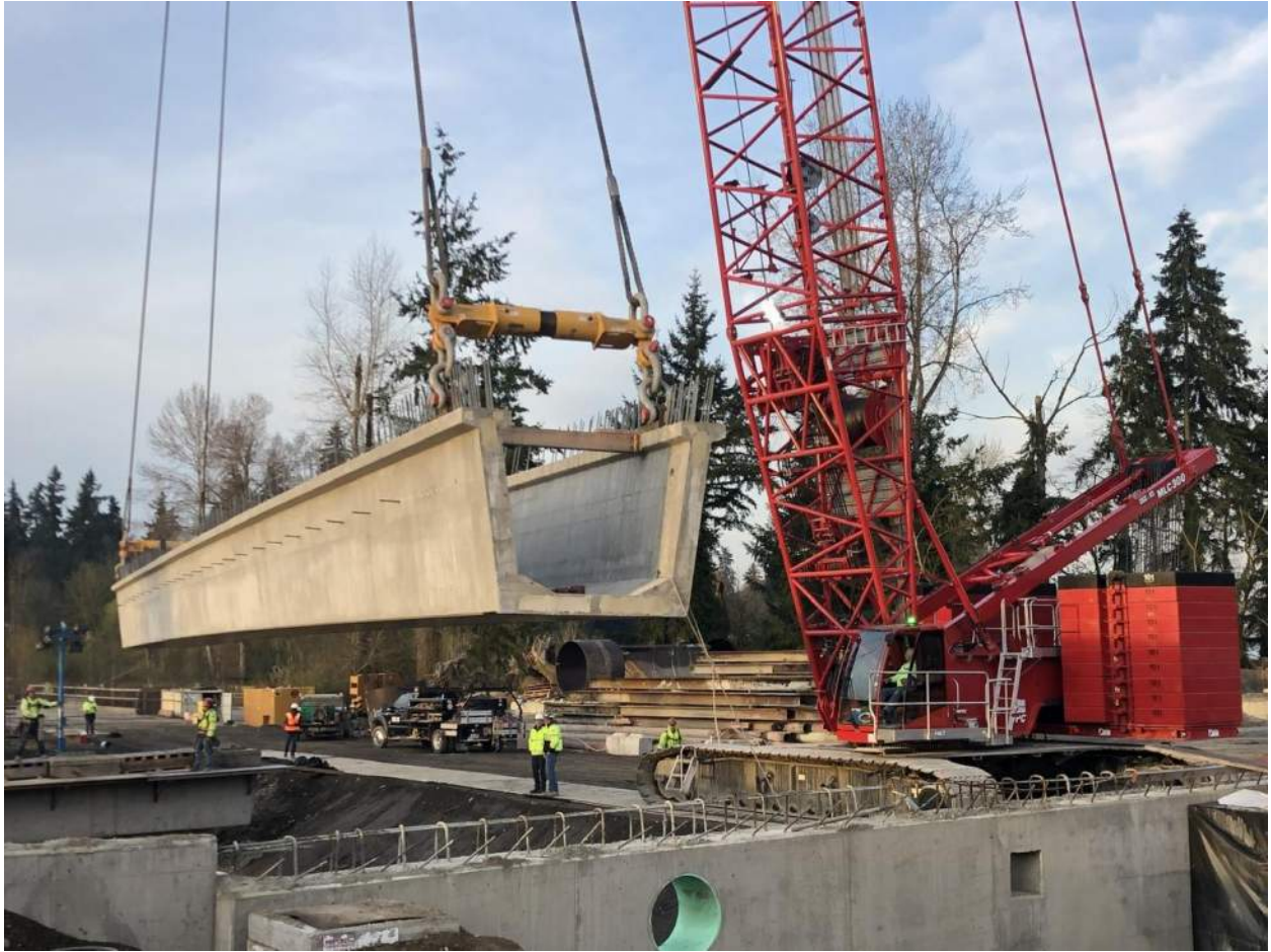
The contractor uses the crane to carefully set each bridge girder on temporary supports at the piers on either side of each span.
