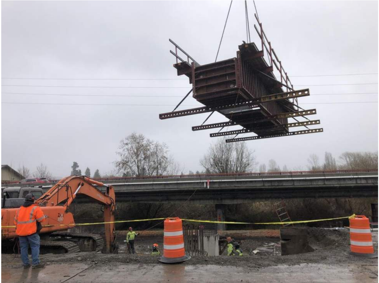
The contractor uses a crane to 'pick' and 'fly' and place the pier crossbeam formwork on top of the bridge columns.
