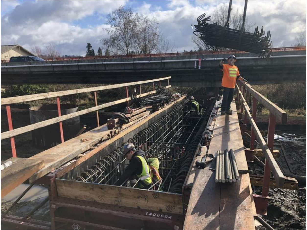
A crane flies bundles of rebar up to the crossbeam formwork for building the crossbeam rebar cage.
