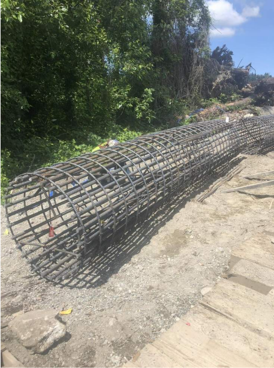
Crews assemble smaller diameter rebar cages for the reinforcement of the bridge columns.
