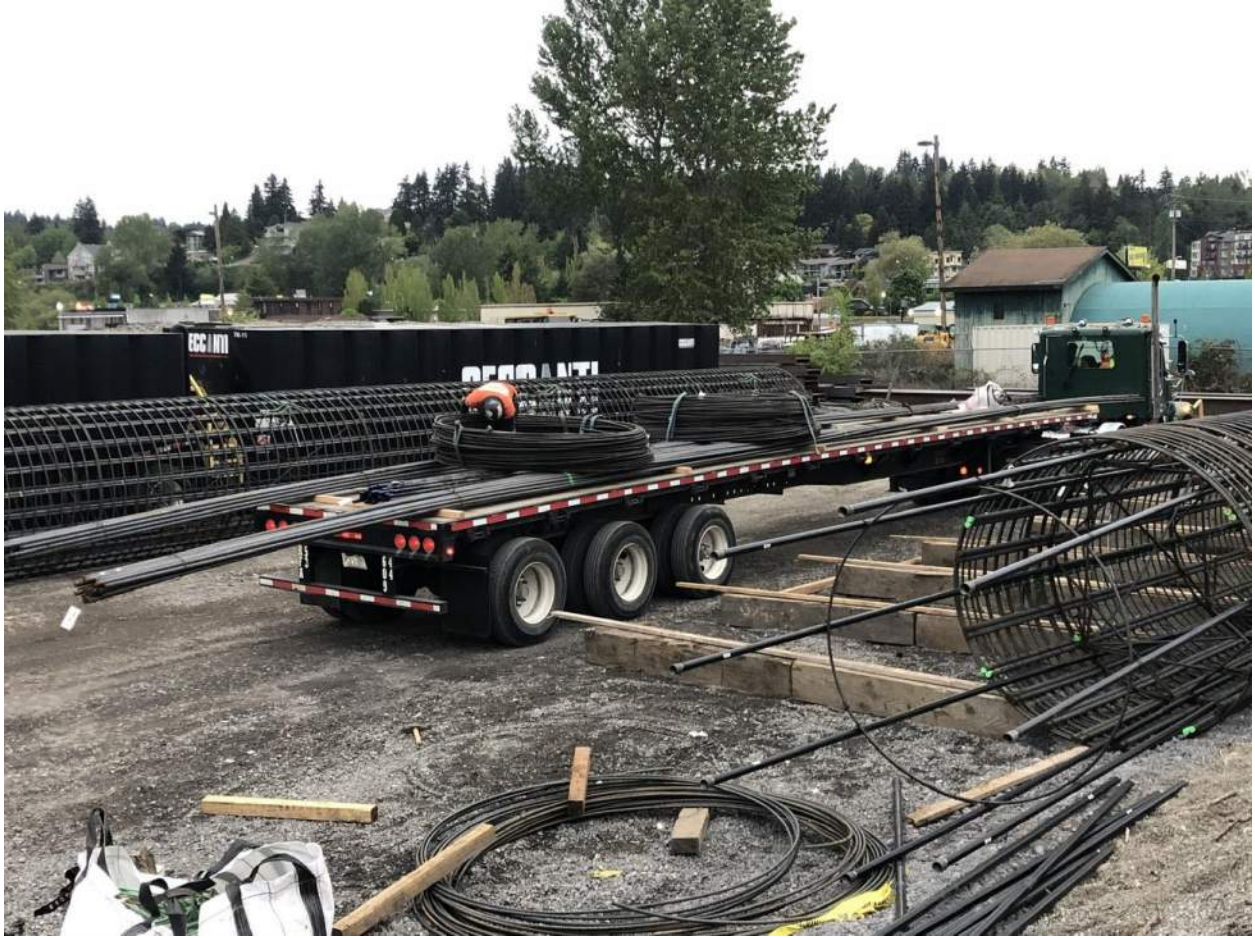
Rebar is delivered onto the project site for building the bridge foundation shaft rebar cages.
