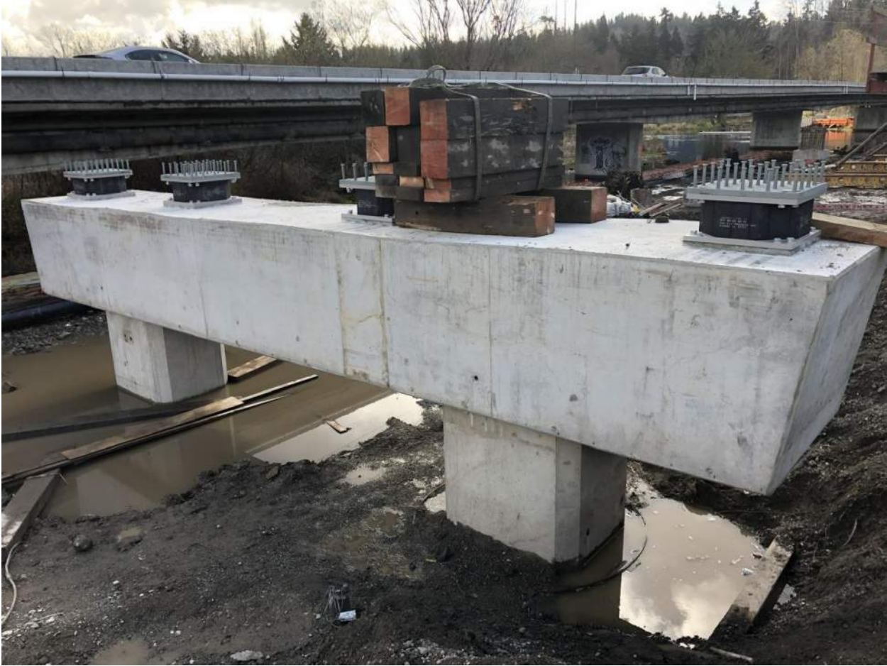
Once the crossbeam concrete has hardened, the outer steel formwork is removed.
