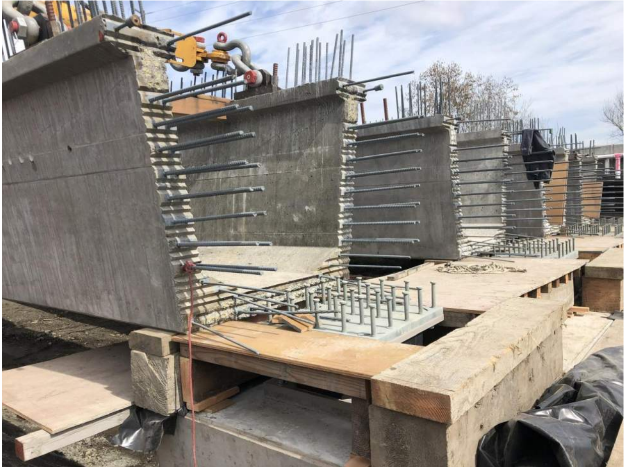
The ends of the girders at each interior pier rest on temporary wood blocking until the remainder of the spans are in place and more concrete is poured to make the structure continuous.
