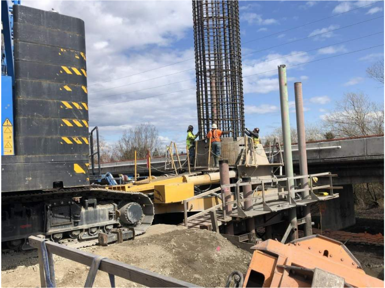
The finished shaft rebar cage (steel reinforcement) is lowered into the fully excavated shaft hole.
