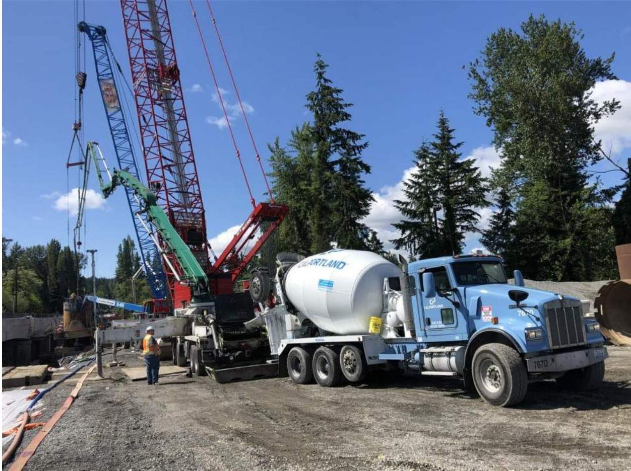
The shaft is filled with concrete from a concrete truck (blue and white) to a pump truck (green) through a pipe into the bottom of the shaft hole.
