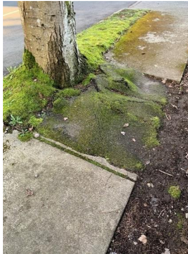
Figure 56. Root system of the subject tree is severely impacting the existing sidewalk.
