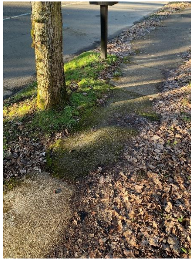
Figure 35. Significant damage to the sidewalk from the root system of the subject tree.
