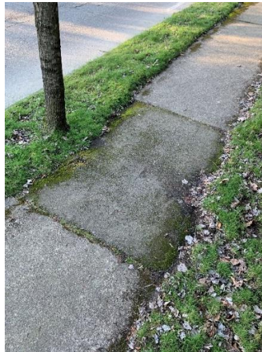
Figure 20. Minor damage to the existing sidewalk.
