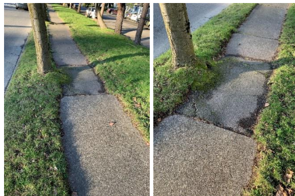
Figure 13. Trunk and roots causing uplift and damage to the existing sidewalk.
