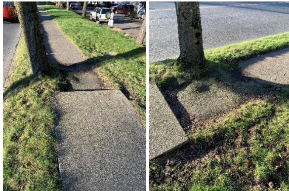
Figure 14. Significant damage caused by trunk and root system.
