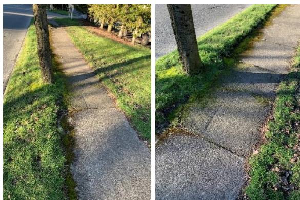
Figure 16. Minor damage caused by the trunk and root system.
