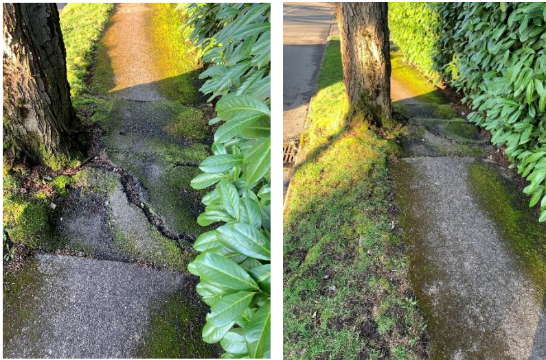
Figure 32. Major damage to the existing sidewalk caused by the shallow rooting system and trunk.
