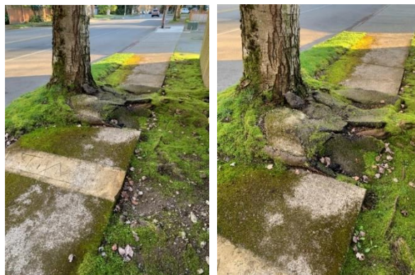
Figure 58. Severe impact to the existing sidewalk caused by the root system of the subject tree.
