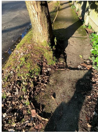
Figure 38. Significant damage to the existing sidewalk creating a hazard.
