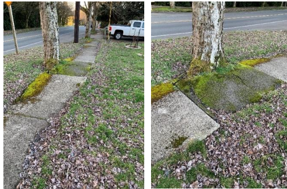
Figure 63. Severe impact to the existing sidewalk caused by the shallow root system.
