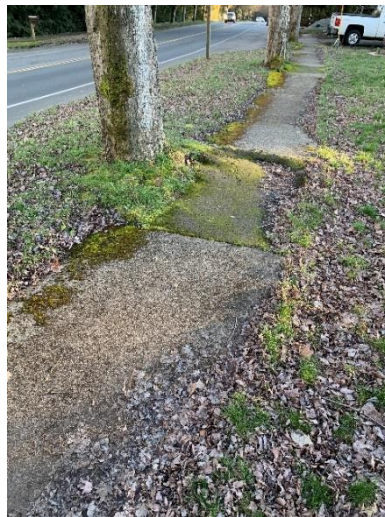
Figure 62. Significant impact to the existing sidewalk due to the root system of the subject tree.
