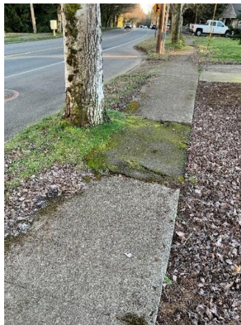
Figure 61. Significant impact to the existing sidewalk caused by the root system of the subject tree.
