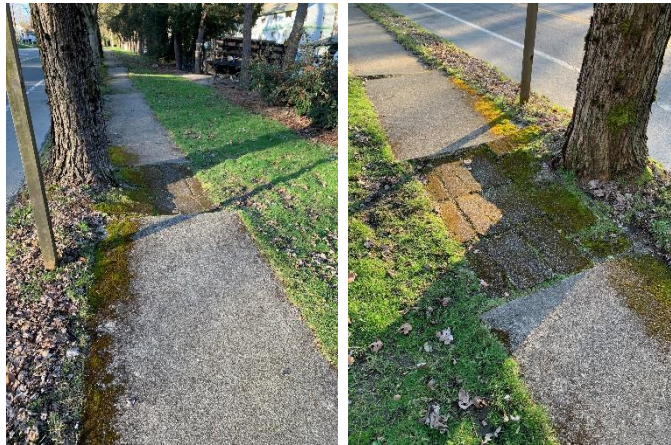
Figure 5. Trunk of Tree #104 directly impacting the existing sidewalk pavers.
