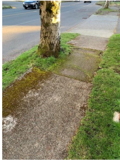
Figure 60. Minor impact on the existing sidewalk due to the root system.
