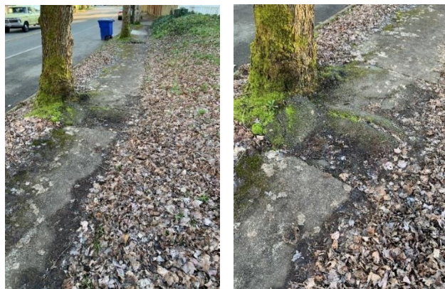
Figure 52. Root system severely impacting the existing sidewalk creating a hazard for pedestrians.
