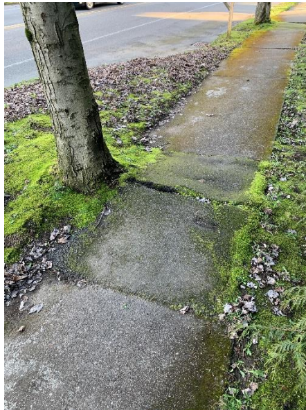
Figure 29. Significant damage to the existing sidewalk.
