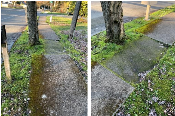
Figure 30. Significant damage to the existing sidewalk from the shallow root system.
