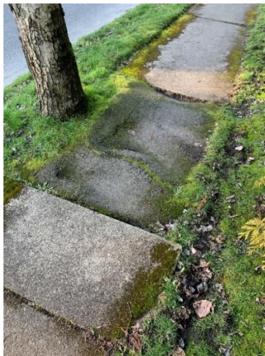
Figure 19. Significant damage caused by the trunk and root system of Tree #118.
