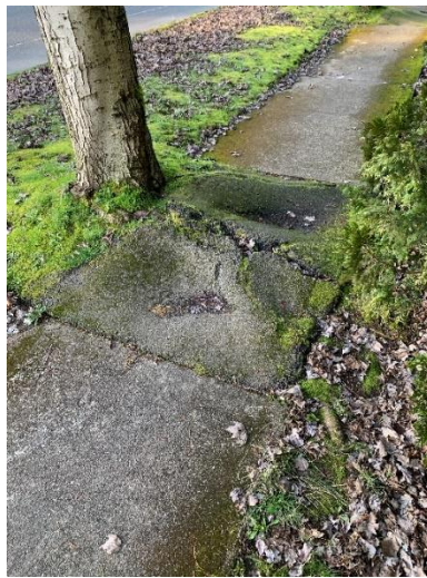
Figure 27. Significant damage to the existing sidewalk from the root system.
