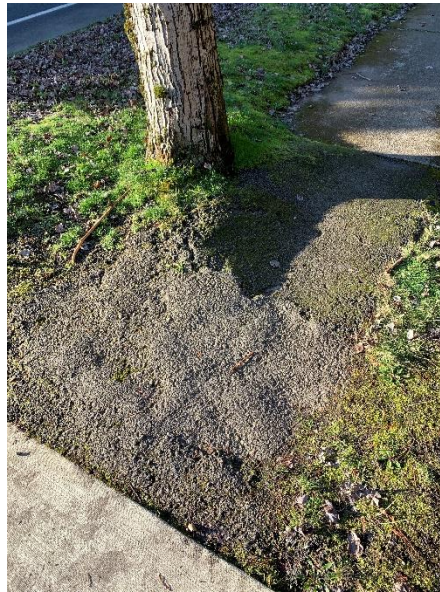
Figure 26. Major damage to the existing sidewalk from the shallow root system.
