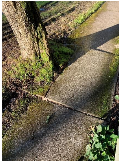
Figure 39. Minor uplift of the existing sidewalk from surface roots.
