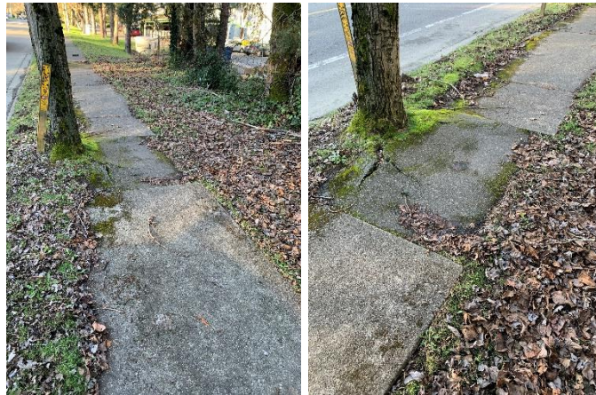
Figure 8. Trunk of Tree #107 abutting against the existing sidewalk causing significant damage.
