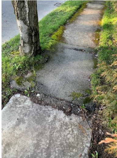
Figure 18. Minor damage to the sidewalk caused by the trunk and the root system.
