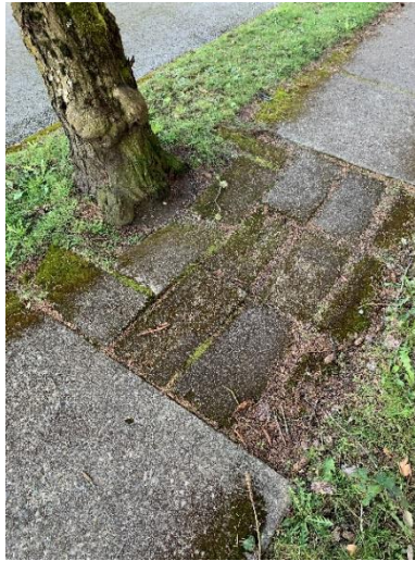
Figure 47. The subject tree is in Poor condition and should be removed and replaced with a more suitable species.
