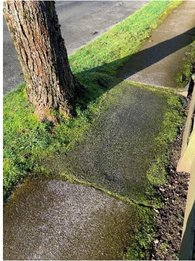
Figure 42. Very minor damage to the existing sidewalk from the trunk and surface roots.
