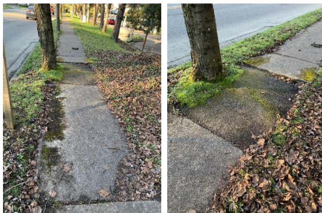
Figure 9. Trunk immediately abutting against the existing sidewalk causing significant damage.
