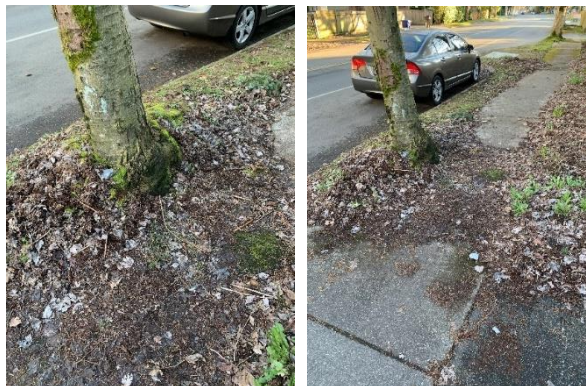
Figure 55. Root system of the subject tree is severely impacting the existing sidewalk.
