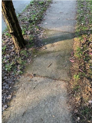
Figure 4. Tree #103 whose trunk is abutting against the existing sidewalk, resulting in minor uplift.
