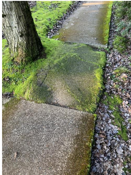
Figure 28. Significant damage to the existing sidewalk.
