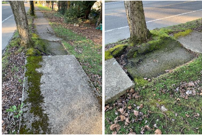
Figure 7. Major damage to the existing sidewalk from the shallow root system of Tree #106.
