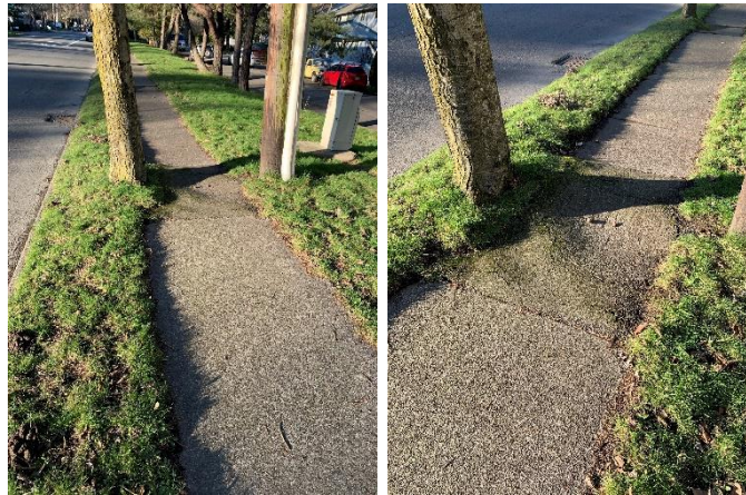
Figure 12. Trunk of Tree #111 already abutting against the sidewalk with no room within the planting strip.
