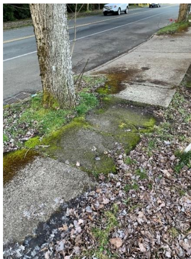
Figure 64. Severe impact to the existing sidewalk caused by the shallow root system.
