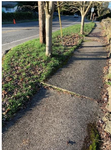
Figure 49. Minor uplift of the existing sidewalk due to surface roots of the subject tree.
