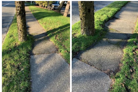
Figure 15. Trunk and root system causing damage to the existing sidewalk.
