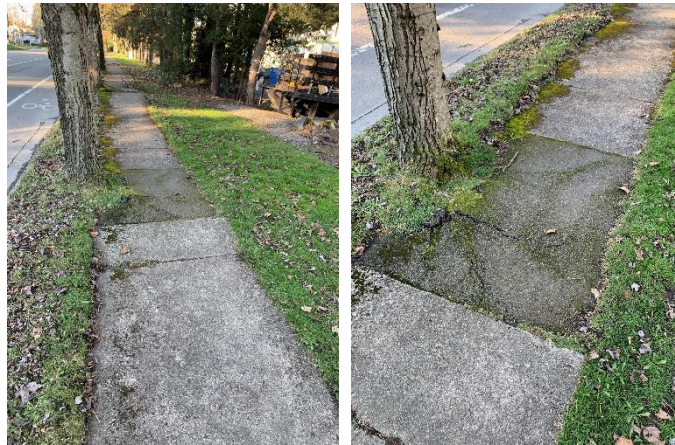
Figure 6. Tree #105 already damaging the newly replaced sidewalk.
