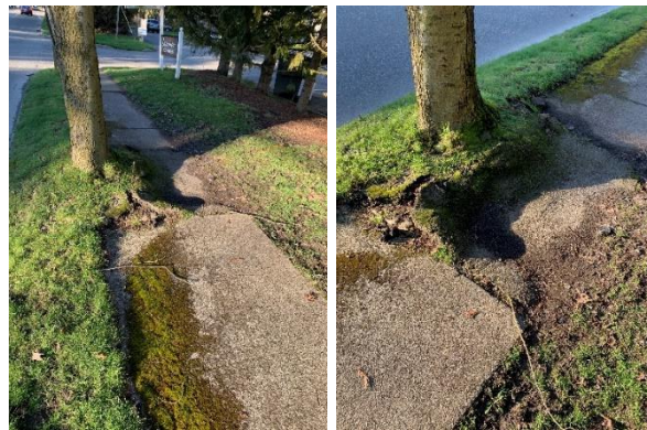
Figure 17. Significant damage caused by the existing tree.
