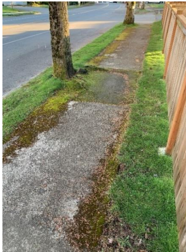
Figure 59. Minor uplift of the existing sidewalk due to the root system.
