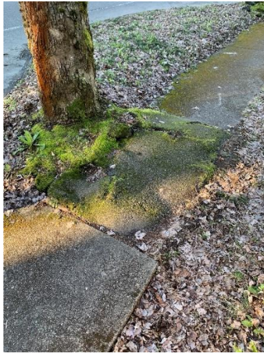
Figure 36. Significant uplift and damage of the existing sidewalk.
