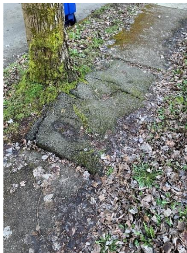
Figure 53. Root system severely impacting the existing sidewalk creating a hazard for pedestrians.
