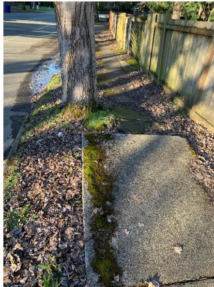
Figure 33. Significant uplift of sidewalk caused by the shallow root system.
