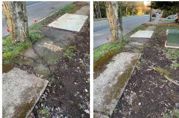
Figure 65. Severe impact to the existing sidewalk caused by the shallow root system of the subject tree.
