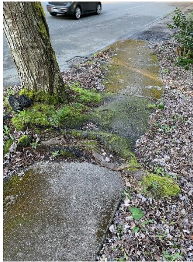
Figure 37. Major uplift and damage to the existing sidewalk from the shallow root system.
