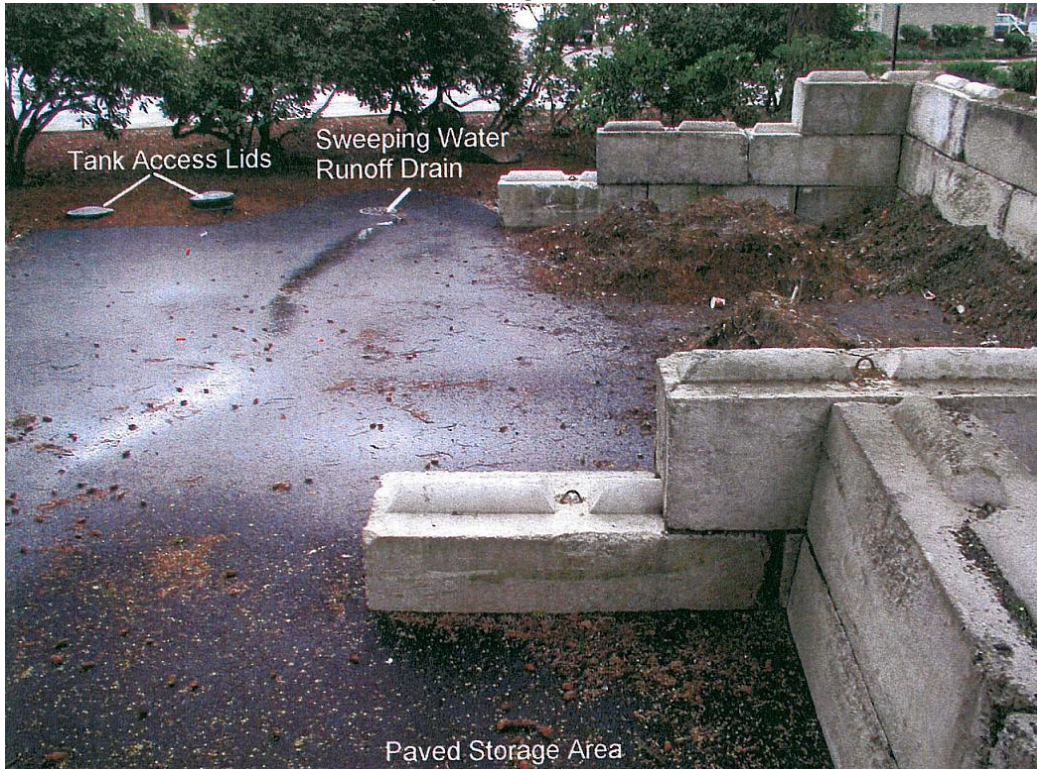
View of facility from north looking south. All surface runoff is collected in drain.
