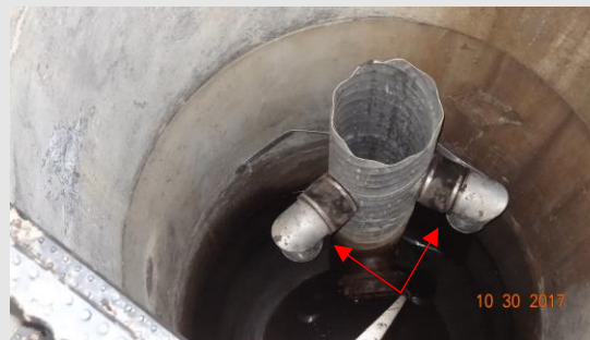
◀ Additional components are frequently added to the basic control structure. Here, there is an additional downturn elbow.
