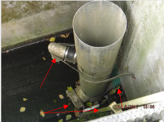
▲ The basic shape of a control structure: a metal or corrugated metal tube (FROP-T), shear gate and rod, outflow pipe at the bottom, a downturn elbow, and an orifice plate welded to the bottom
