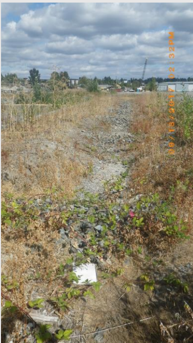
◀ Bad: This ditch has exposed soil and dead vegetation. Maintenance will be needed for this ditch to be effectively filter water
