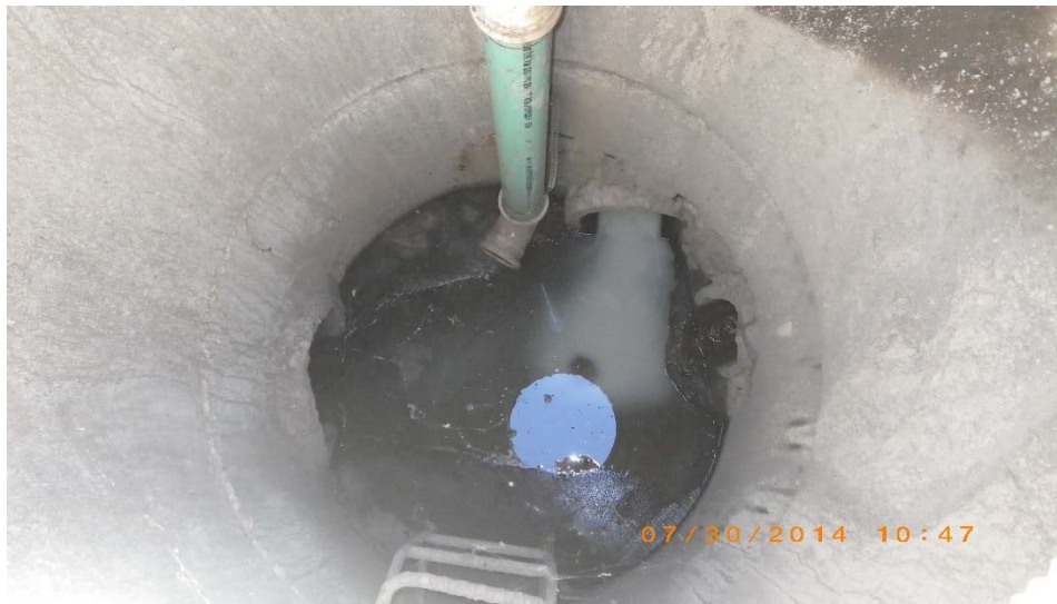
Utilizing field screening techniques during annual MS4 inspections, inspectors are able to identify illicit discharges, such as the one above, for elimination.
