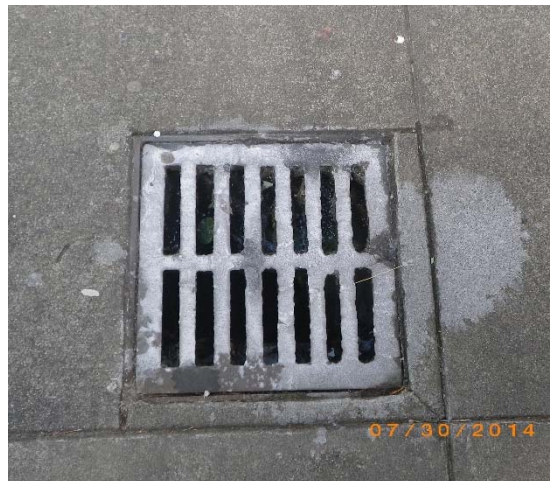
Surface staining is an indicator that inspectors use to identify illicit discharges.
