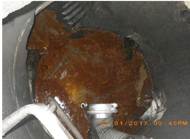
Discharges that pose a threat to human health and the environment may require immediate response.
